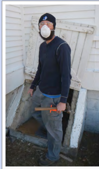
Mark Doperalsky preparing to enter the privy to remove the last of the concrete cap.
